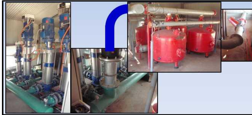
Figure 4: This collage of photos shows a three pump system teamed up with a massive 4 x 48" media filtration system, requiring a flow output 50% in addition to the pump system capacity during backflush, but which was not allowed for. With no pressure sustaining valve, the result was that the pumps and VFD's suffered periodic failure, not to mention the significant field pressure loss during backflush and hence low CU's and DU's to the golf course it served.
