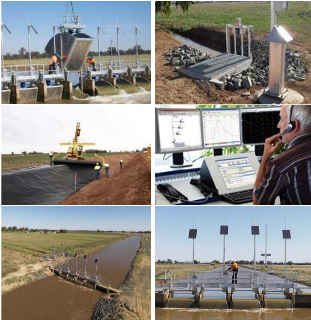
Figure 6 – Modernized Canals in Victoria's NVIRP Project
