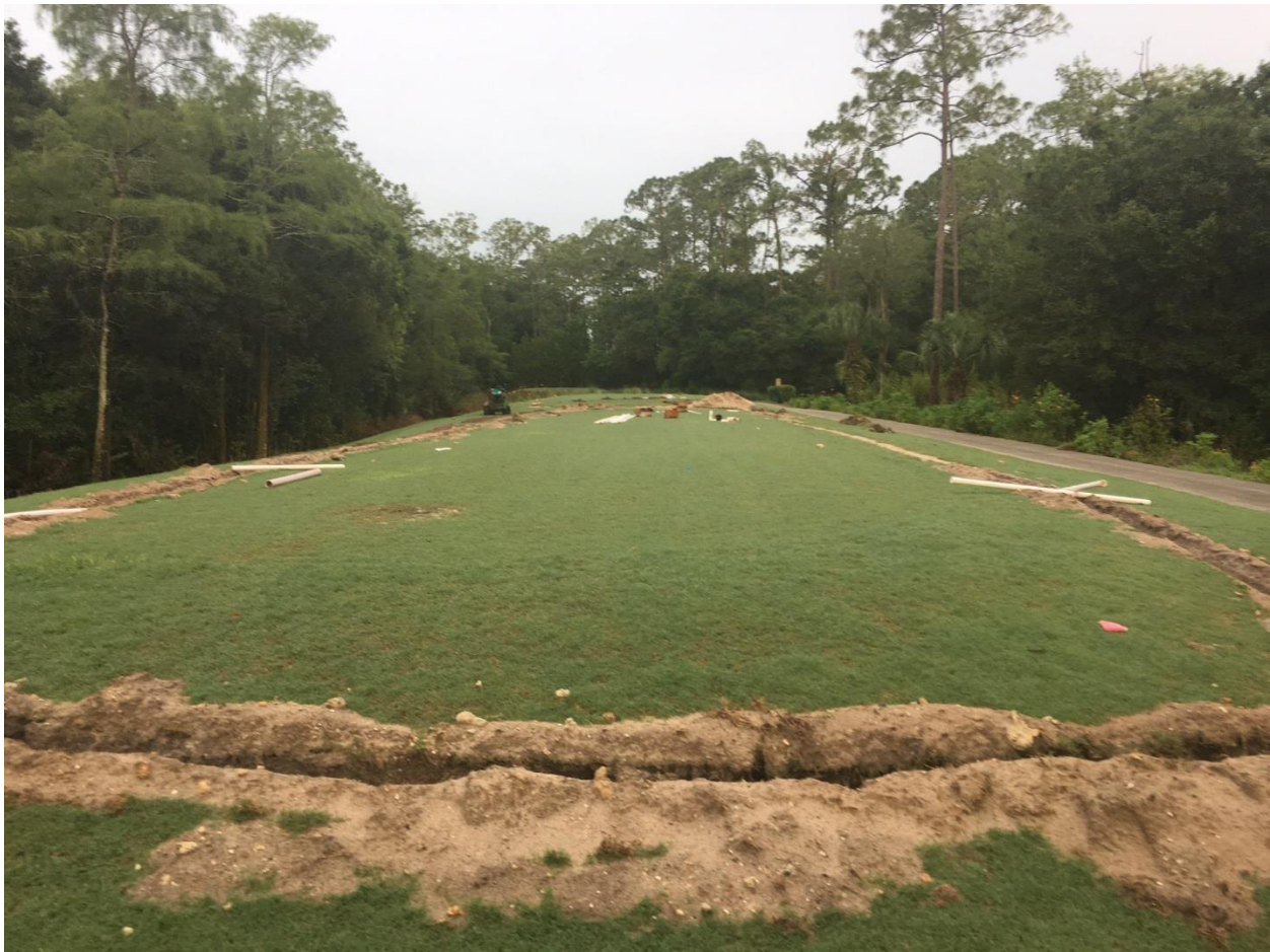
Figure2. Installation of new block-zone design, note the narrow width of the irrigated site
