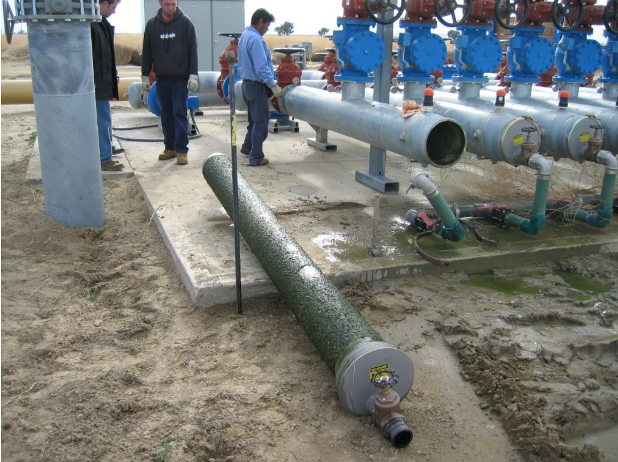
Figure 1. Typical horizontal cylindrical filter with a coarse, perforated stainless steel screen, typically used for sprinkler applications. Algae that passed through the screen can be seen on the downstream side of the screen. The complete screen has been removed from the filter housing. A 4" flush-through (not backflush) valve and hose manifold can be seen for each cylinder.
