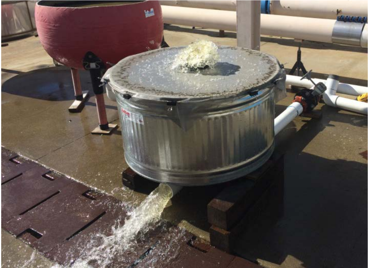
Figure 5. ITRC mushroom screen for cleaning and recirculation of filter backflush water.
