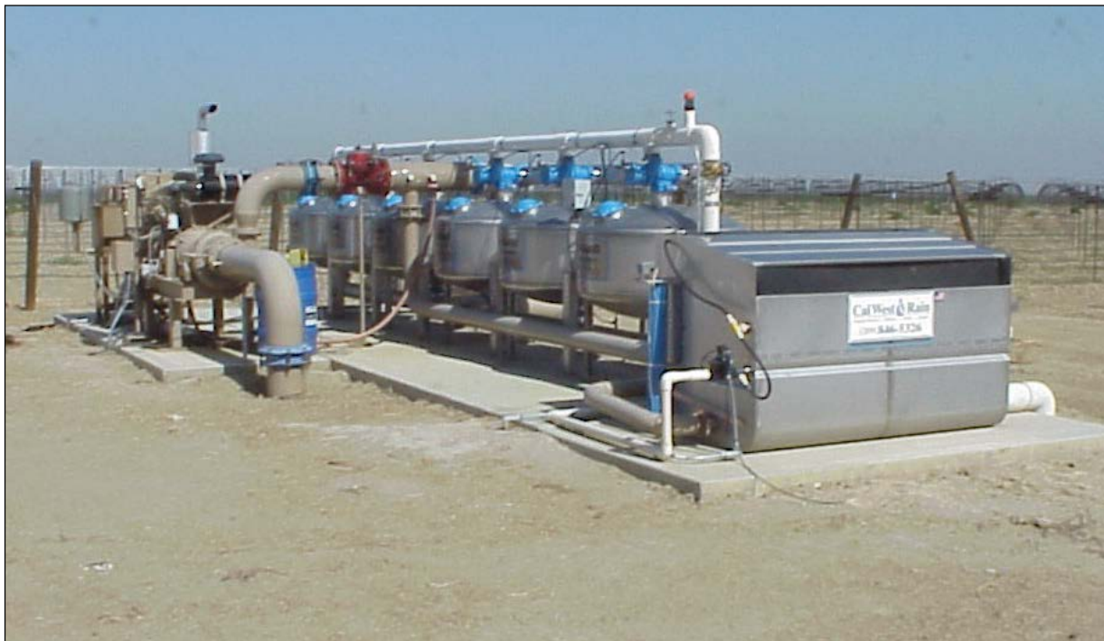
Figure 4. A media tank filtration system that uses a small commercial (FV&C) overflow screen to clean the backflush water before recycling it
