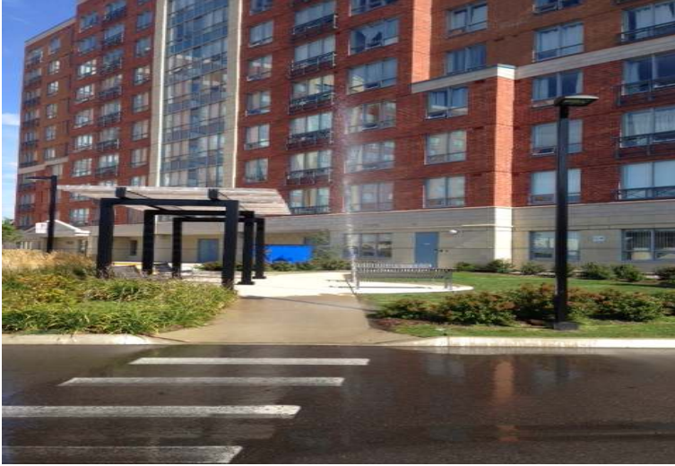
Example of a leak
