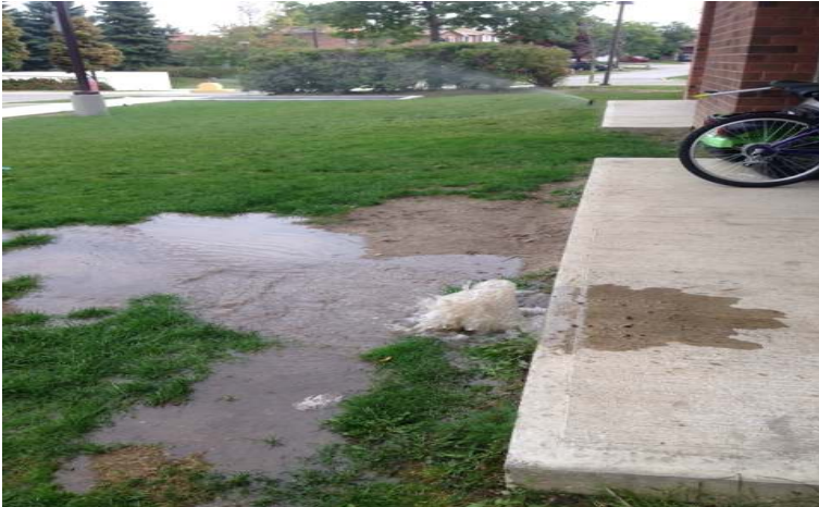
Example of a leak- Some deficiencies are more visible than others.
