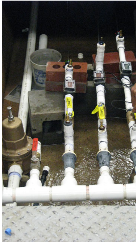
Figure 1. Picture of Pressure Regulator Test Stand, including manifold, pressure regulator, pressure shunt, water meter, pressure shunt and flow nozzle.
