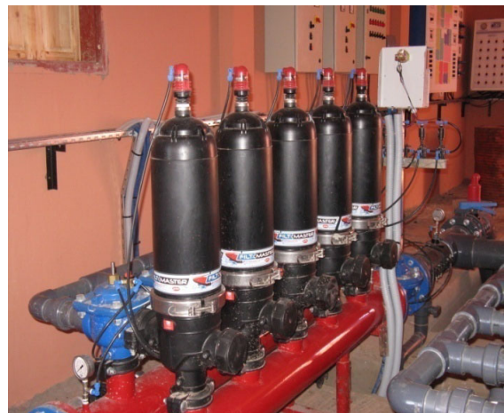
Figure 10. Disk filters. PIT, March 2009
