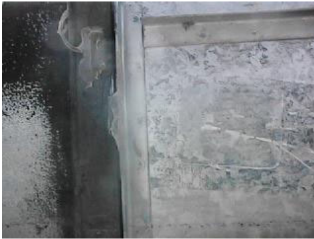
Fig 3. Switch and magnet attached to a slide gate.
