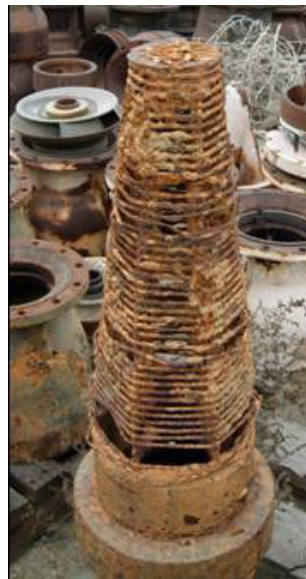
Figure 7. Corroded pump cone screen with missing sections.
