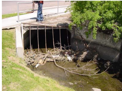
Fig. 5. Upstream side of a bridge where debris has collected (Logan Northwest Field canal)
