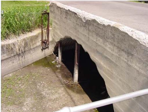
Fig. 2. Culvert inlet and a deteriorated outlet gate (Northwest Field canal)
