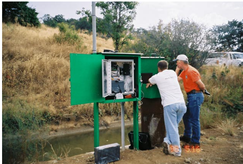
Photograph 4. This view of the site on Talent Canal shows the equipment cabinet containing the data logger and dial-up equipment. The technicians are installing the float well equipment which was used to verify the depths obtained from the pressure transducer in the Starflow instrument.
