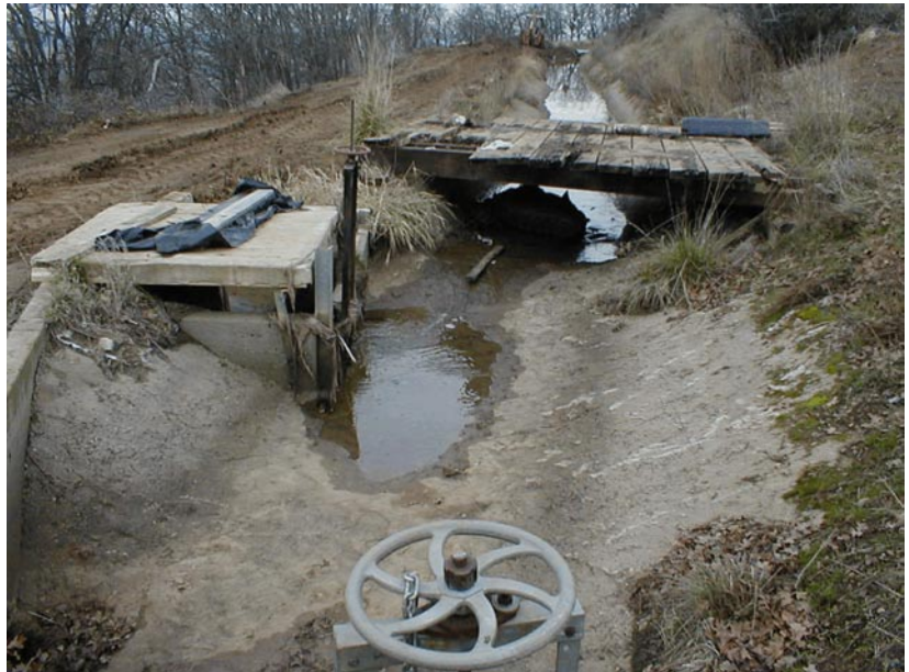
Photograph 2. View is looking upstream in the Talent Canal at the Crooked River Siphon entrance. The StarFlow instrument was installed upstream of the wooden bridge. This section of canal experiences backwater when the spill to the river is not operated. The canal capacity is about 15 cfs.
