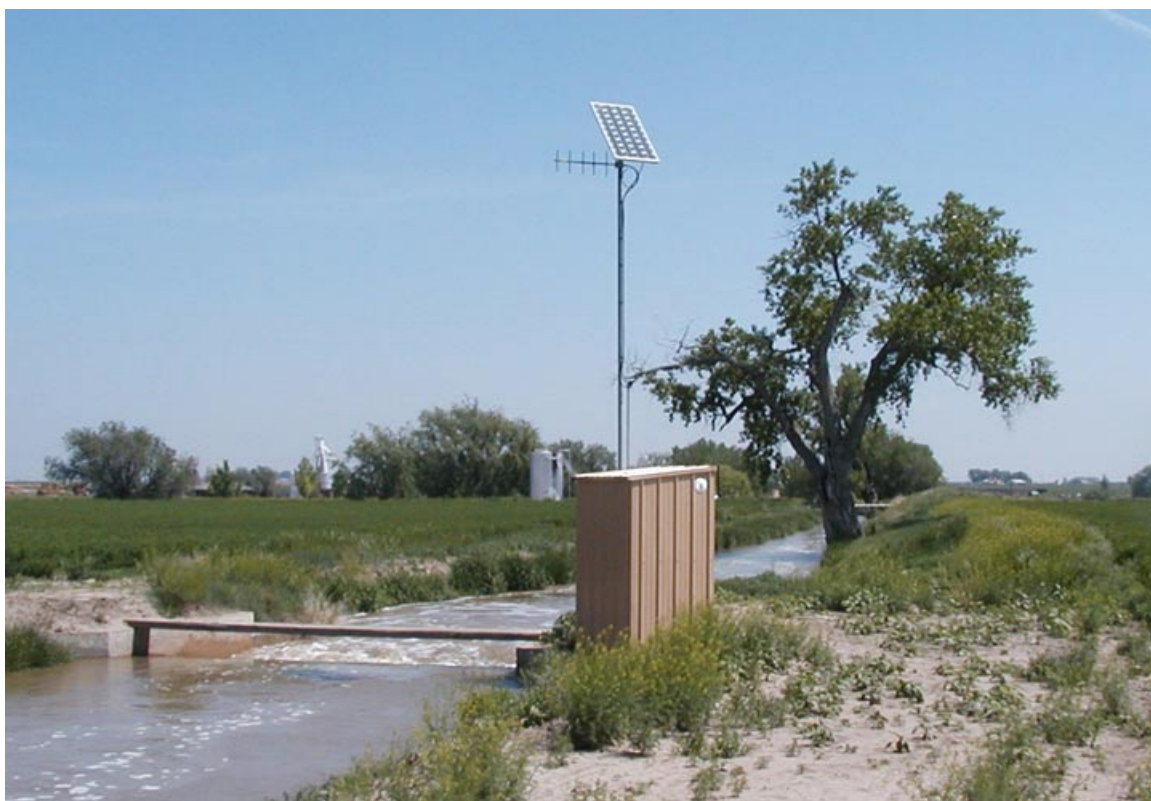
Figure 1. An example of a rated canal section which is remotely monitored using a SCADA system. RTU equipment is 12-volt DC powered from a solar panel that maintains a charge on a battery. Communication with the site is via radio.
