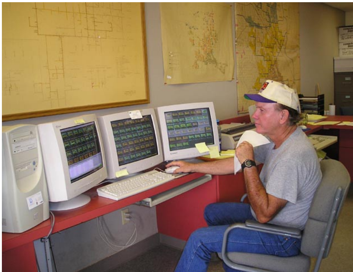
Figure 3. An operator at the Central Arizona Irrigation and Drainage District (CAIDD) near Phoenix monitors primary flows and water surface elevations in the 60-mile canal. This SCADA system was implemented at relatively low cost using affordable RTU equipment and spread spectrum radios for communication.
