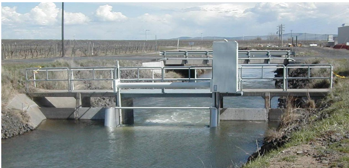
Figure 4. This check structure is controlled by a Langemann gate and control is integrated with a SCADA system. Langemann gates function as a check structure and can be used for flow measurements.
