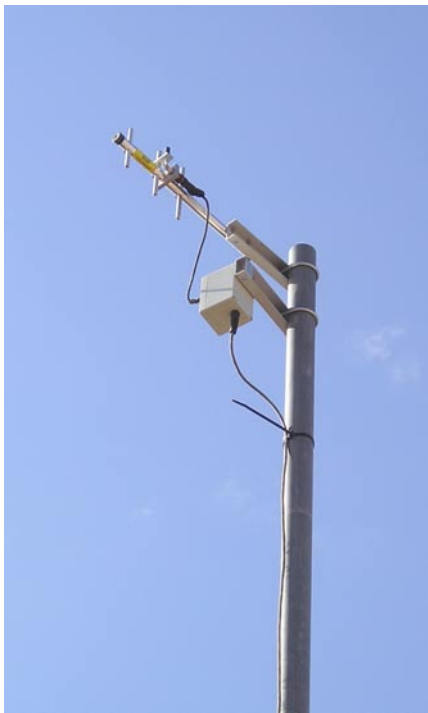
Figure 5. The SCADA system at Central Arizona Irrigation and Drainage District (CAIDD) uses spread spectrum radio which is a relatively new type of radio system that does not require federal licensing. The spread spectrum radio is housed in the white enclosure and the directional antenna shown has a line-of-sight range of approximately 5 miles. The antenna is mounted on a 2-inch galvanized steel pipe.
