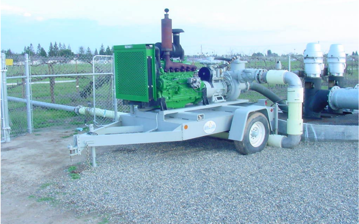
Figure 3 Portable pumping plant. Note the water meter is visible in the 8 inch mainline just outside of the security fence.
