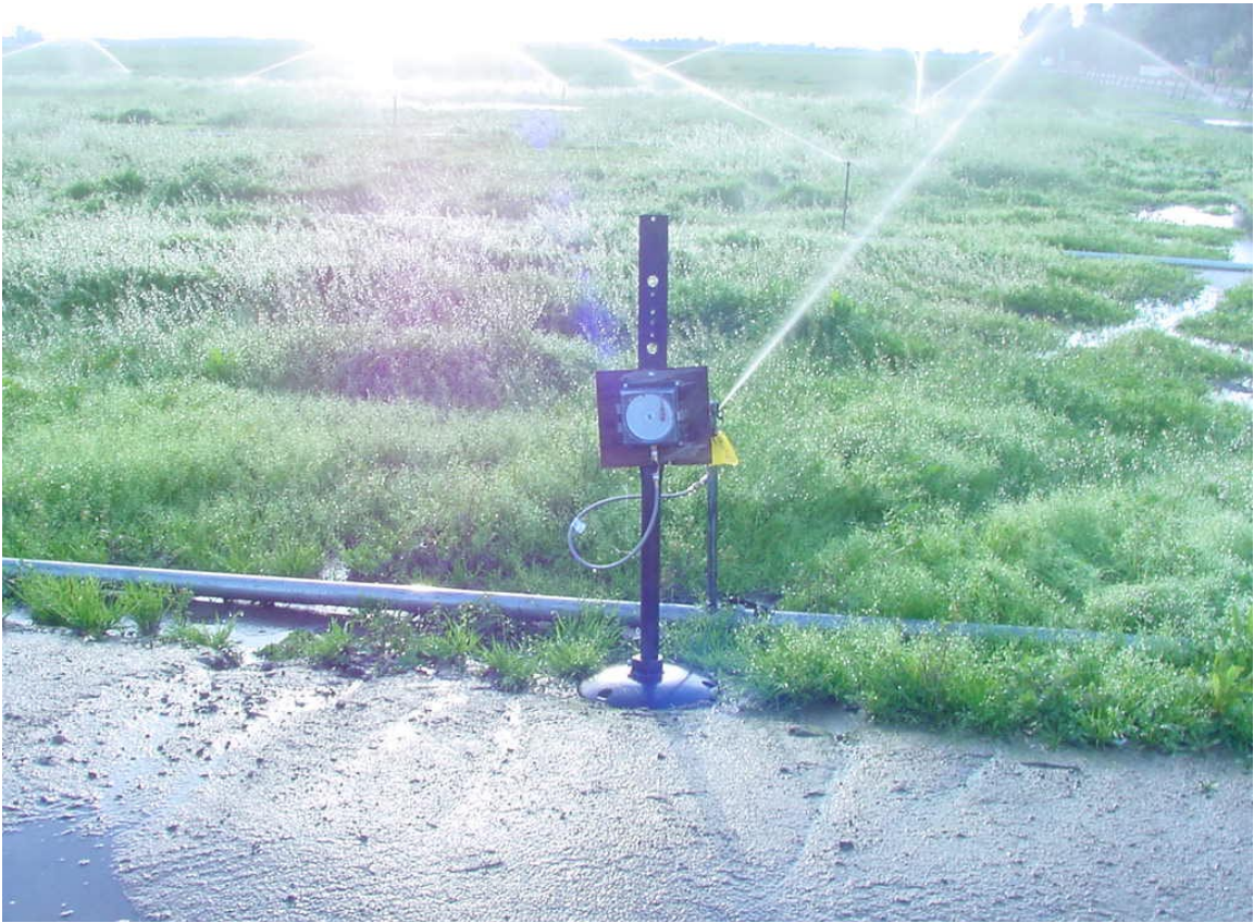
Figure 5 Recording pressure gauge located on the second from the end sprinkler.
