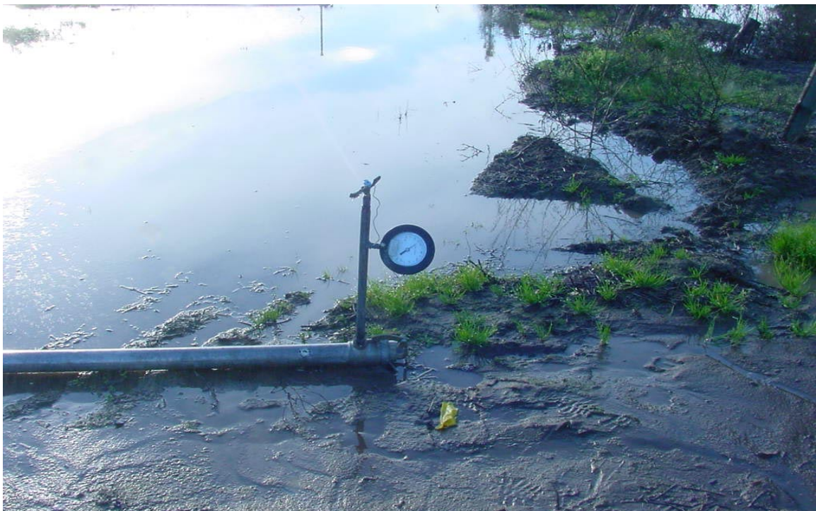
Figure 4 Pressure gauge mounted on a riser at the end of the lateral.
