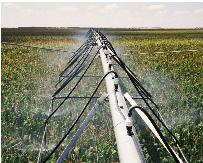
Fig. 3: Pressure regulators installed upstream of drop hoses.
